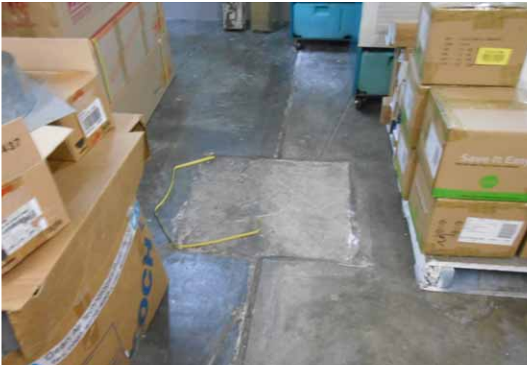
Photo 28 - Replaced square concrete areas noted
