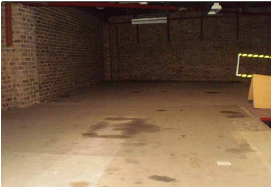
Photo 24 - Minor staining of timber observed in raised storage area
