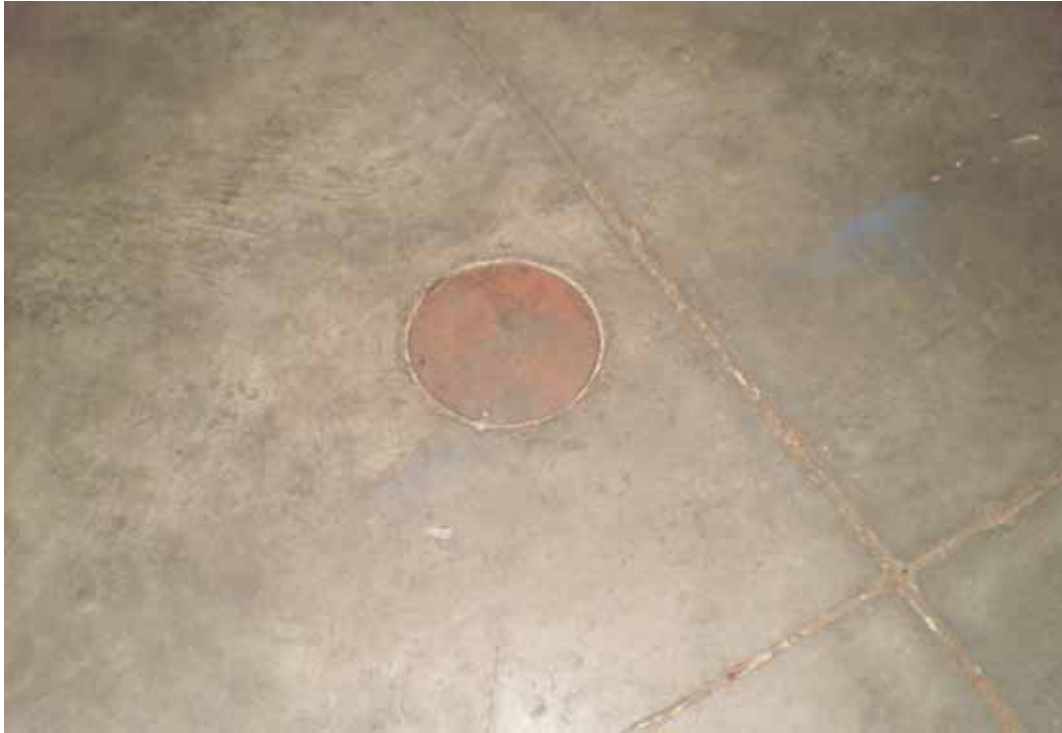
Photo 25 - Round metal cover for unknown pipework
