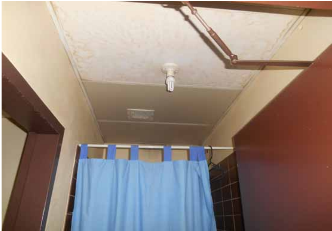
Photo 9 - Potential asbestos-containing roof panels in bathroom area
