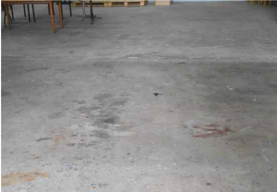
Photo 33 - Minor staining on concrete area of training facility
