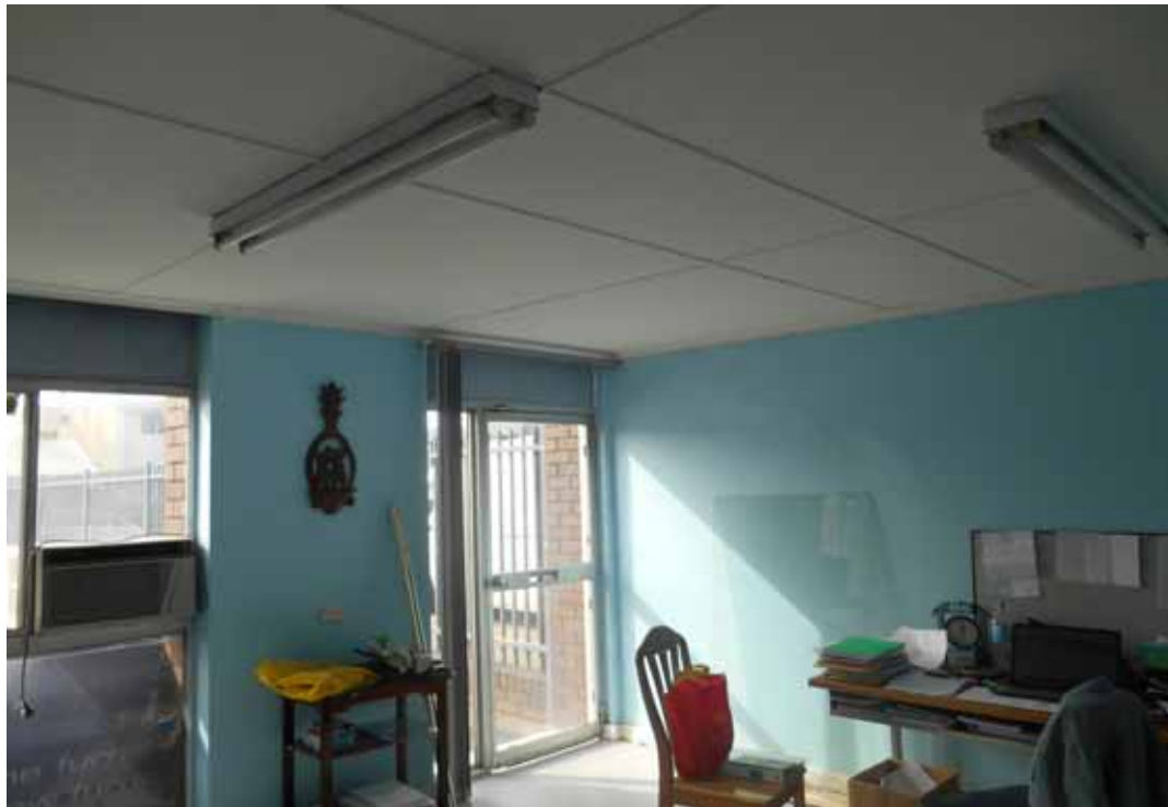
Photo 14 - Potential asbestos-containing FCS roof
